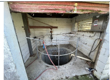
Rangiatea Pump Station
