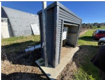
Harpers Ave Pump Station
