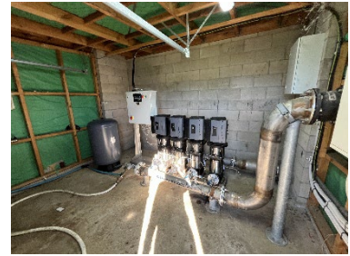
Mckenzie Ave Booster Station
