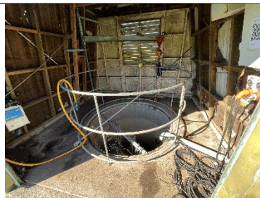
Cedric Smith Pump Station
